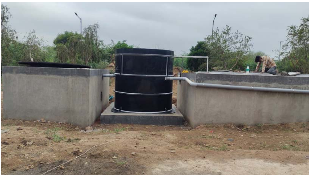
Picture above: Mars 5000 plant implemented at CURAJ
