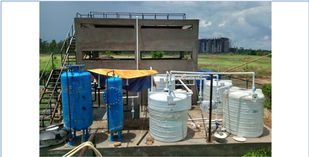
Overview of the implementation area 1.1 – Pilot scale electrically conductive biofilter
